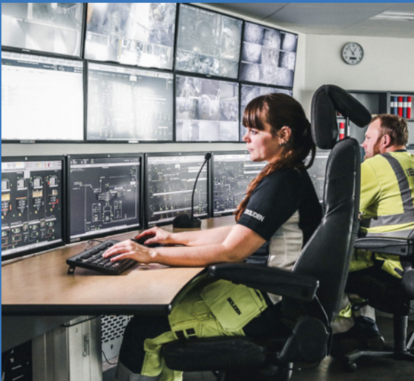
Control room, Garpenberg mine, Sweden (Credit: Boliden)
